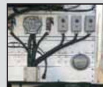
Electrical System Options
